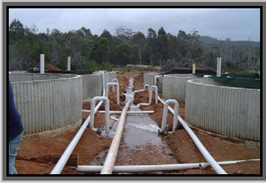
Water reticulation system (Photo: Don Defenderfer)
